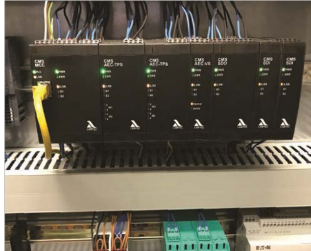
CMS modules installed in the control cabinet.
